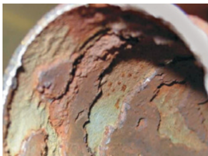
Corrosion in the form of rust and pipe-scale
